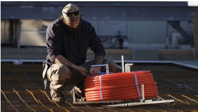
Installing PEX to wire mesh using an automatic tying machine enabled the large job to go quickly. Photo by Todd Plitt
